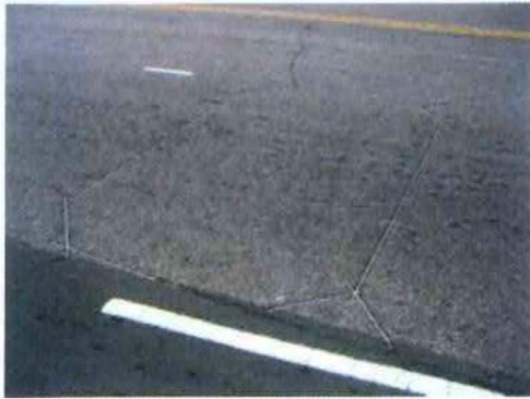
Figure 3-2. Photograph of vehicle detector loop in pavement
