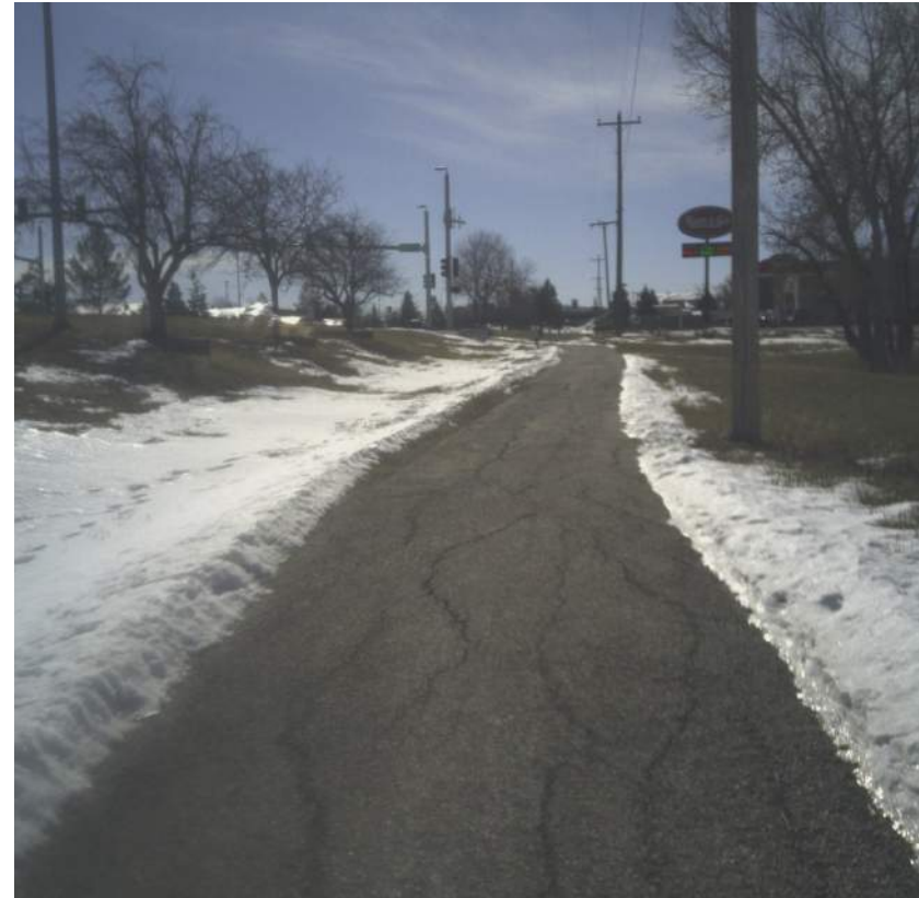
Cracking on asphalt sidepath in Gillette
