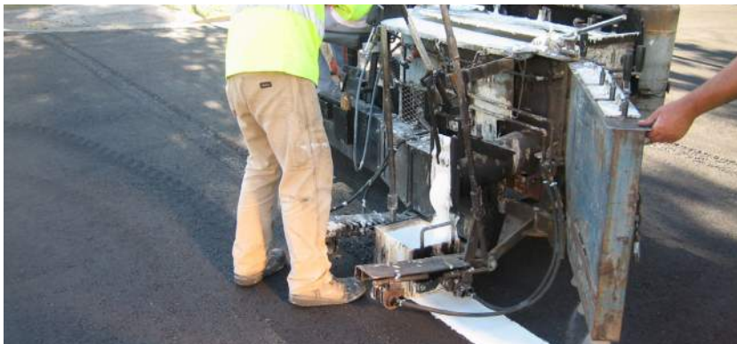
Restriping shoulder is typically necessary once a year in places that receive significant snowfall.
