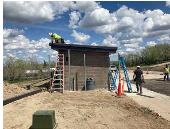
Kliver Road PRV Building
