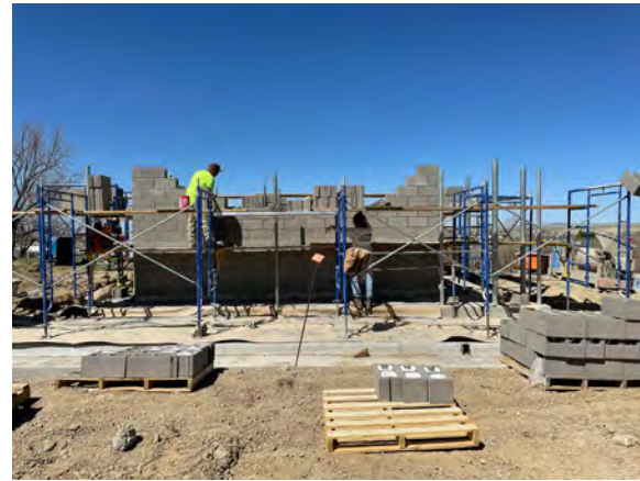
Kliver Road PRV Building
